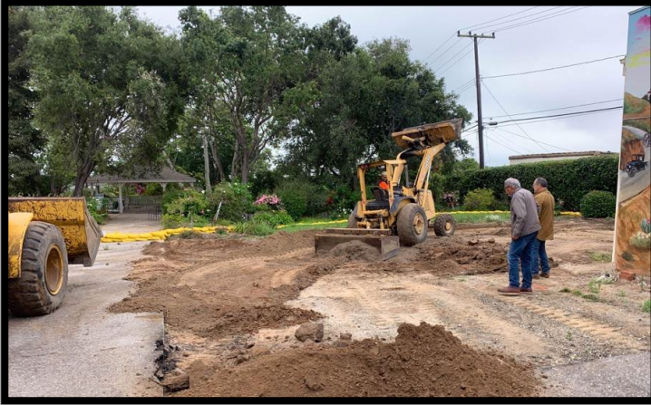
Above: May 22, 2023 – Early in the construction the new building foundation pad begins preparation for compaction.
