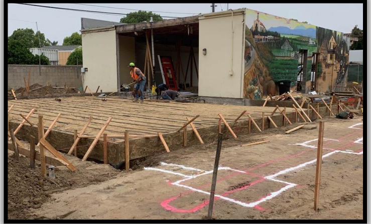
Above: June 11, 2024 – The new building foundation pad is framed, rebar in place and ready for concrete to be poured.
